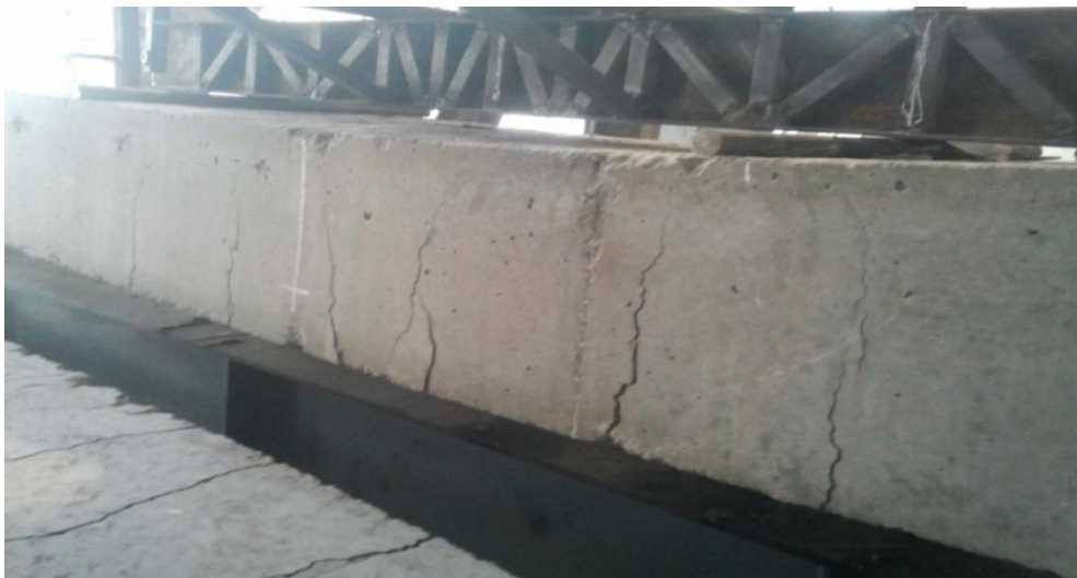
Fig –4.4 Crack Pattern of Controll Specimen 02 (FDB 02)
