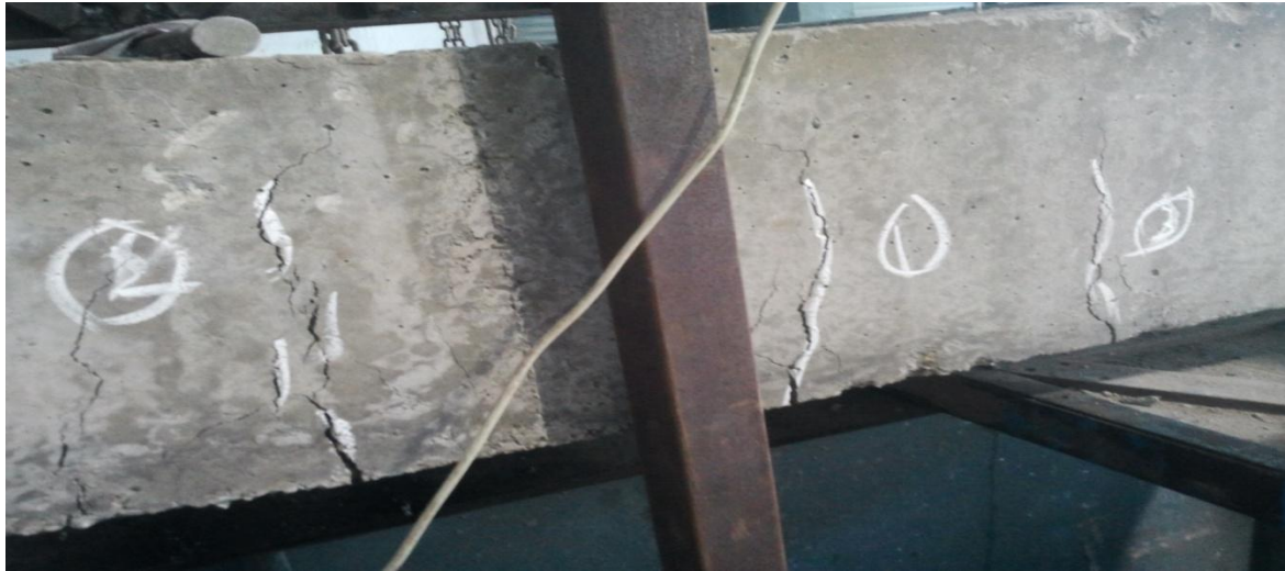
Fig-4.1 Crack Pattern of Control Beam 01 (FDB 01)
