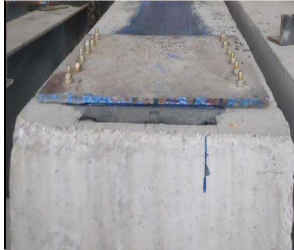
Fig-3.9 Fixing of Fixed End Plate at One End With the Help of Fastner
