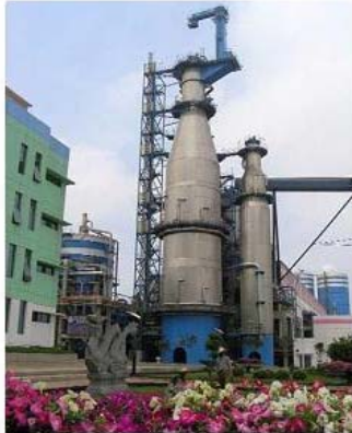
Continuous Kraft digester of duplex stainless steel grade 2205, Hainan Jinhai Pulp & Paper Co. Ltd., China
