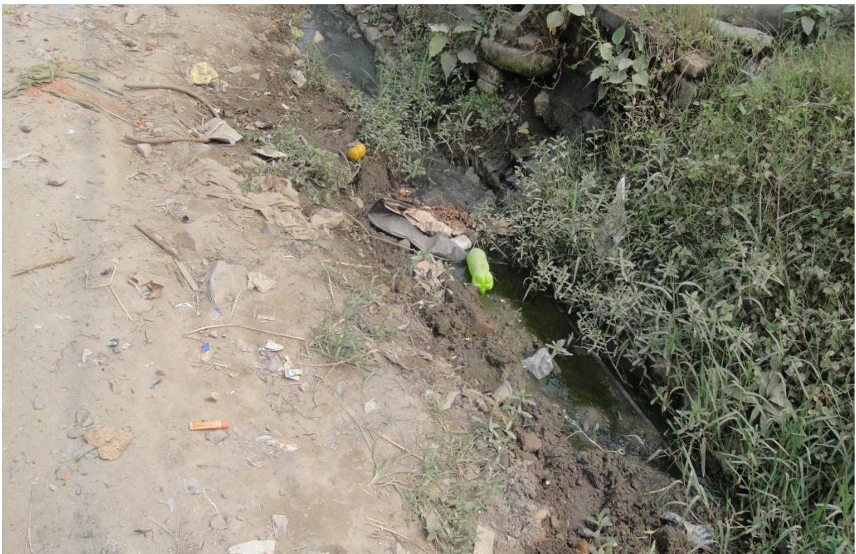
Fig 3.15 Improper Drains along the Project Highway
