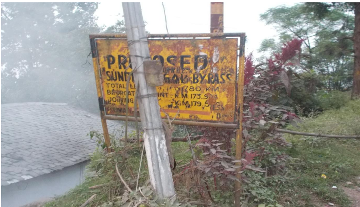
Fig 3.13 Bad Condition of the sign & informatory boards through out the existing highway.
