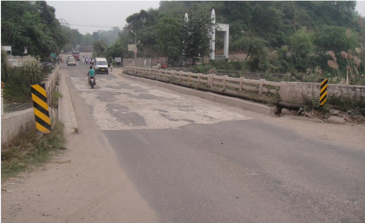
Fig 3.4 Minor Bridge with Poor riding quality & inadequate width
