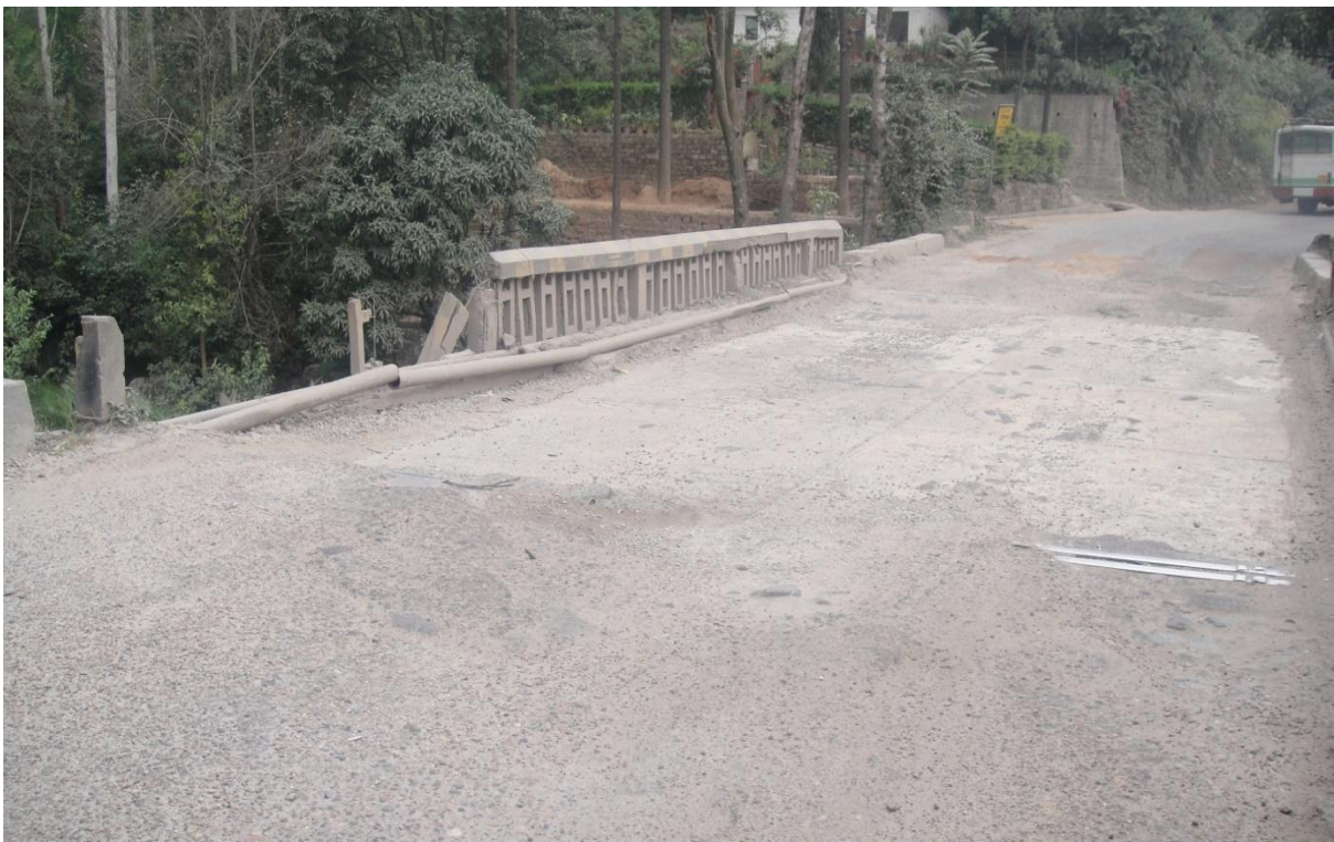
Fig 3.9 Very Poor Road Safety Aspects on the existing two lane highway
