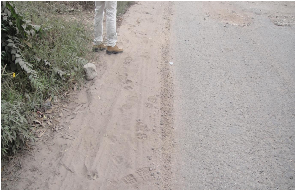
Fig 3.5 Loose Earthen Shoulders all along the existing project highway NH-21
