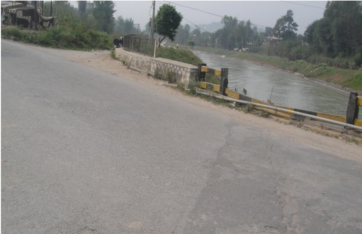
Fig 3.18 Damaged parapets along the existing Highway.
