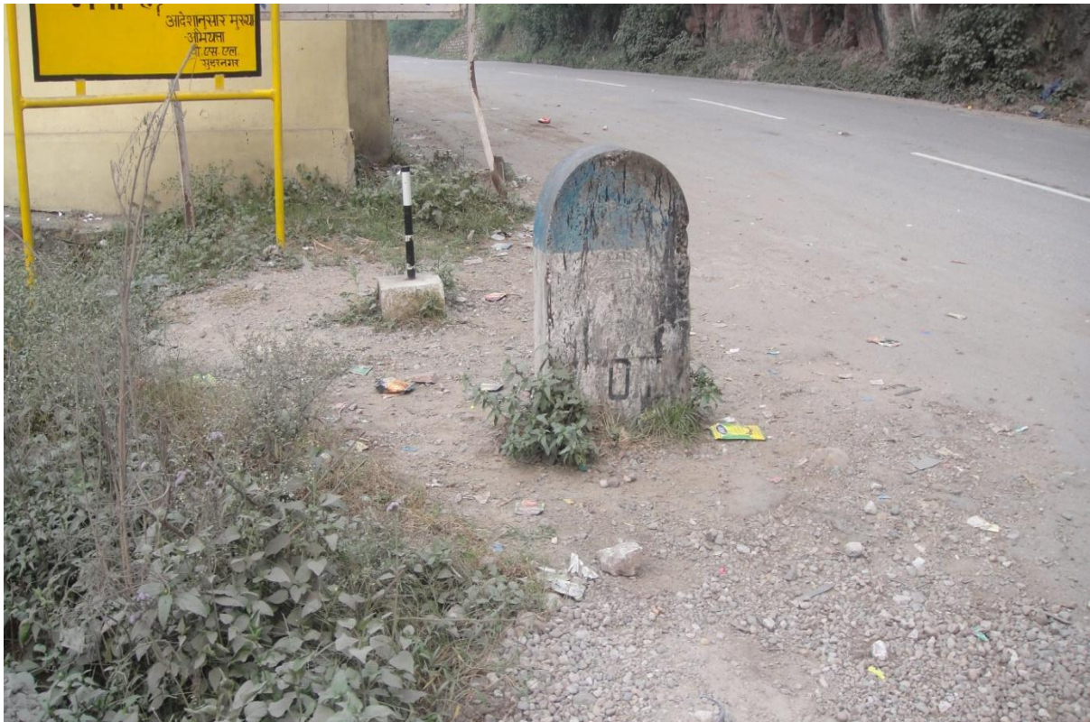
Fig 3.12 Very bad condition of km stone along the old alignment
