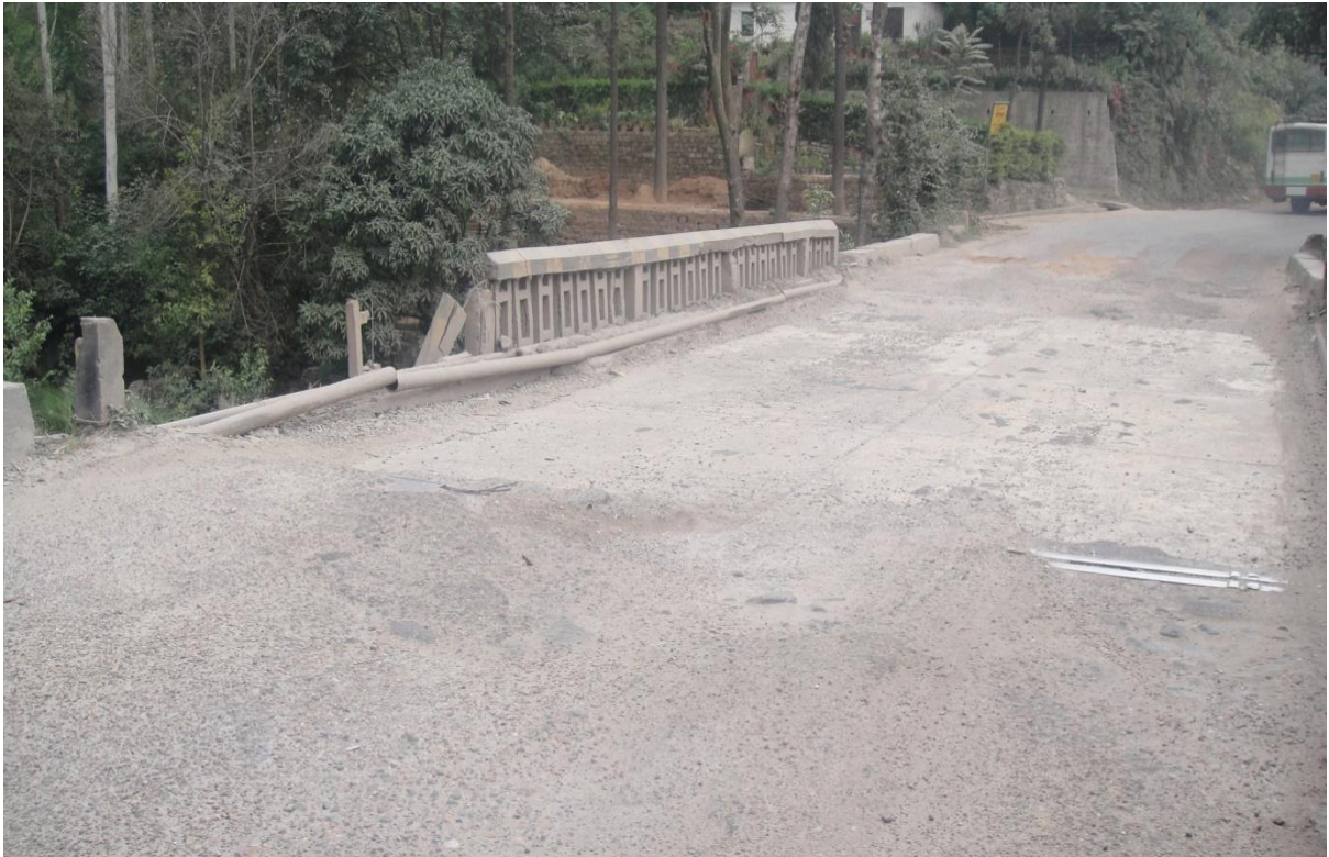
Fig 3.14 Very Poor Road Safety Aspects on the existing two lane highway
