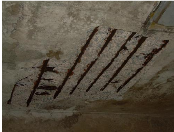
(C) Corrosion in slabs
