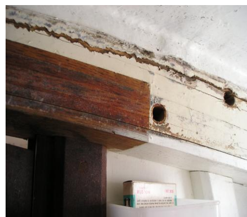
(b) Corrosion of beams
