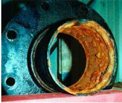
Fig. 2.8 Corrosion on a metal ring due to Sulfur Oxidizing bacteria
