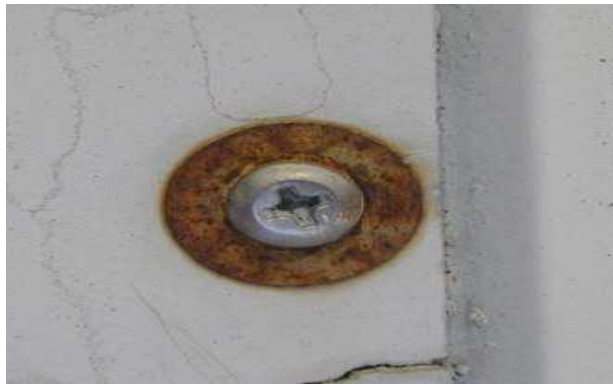
Fig. 2.7 Galvanic corrosion on a metal washer ( Autolab application note 16 )
