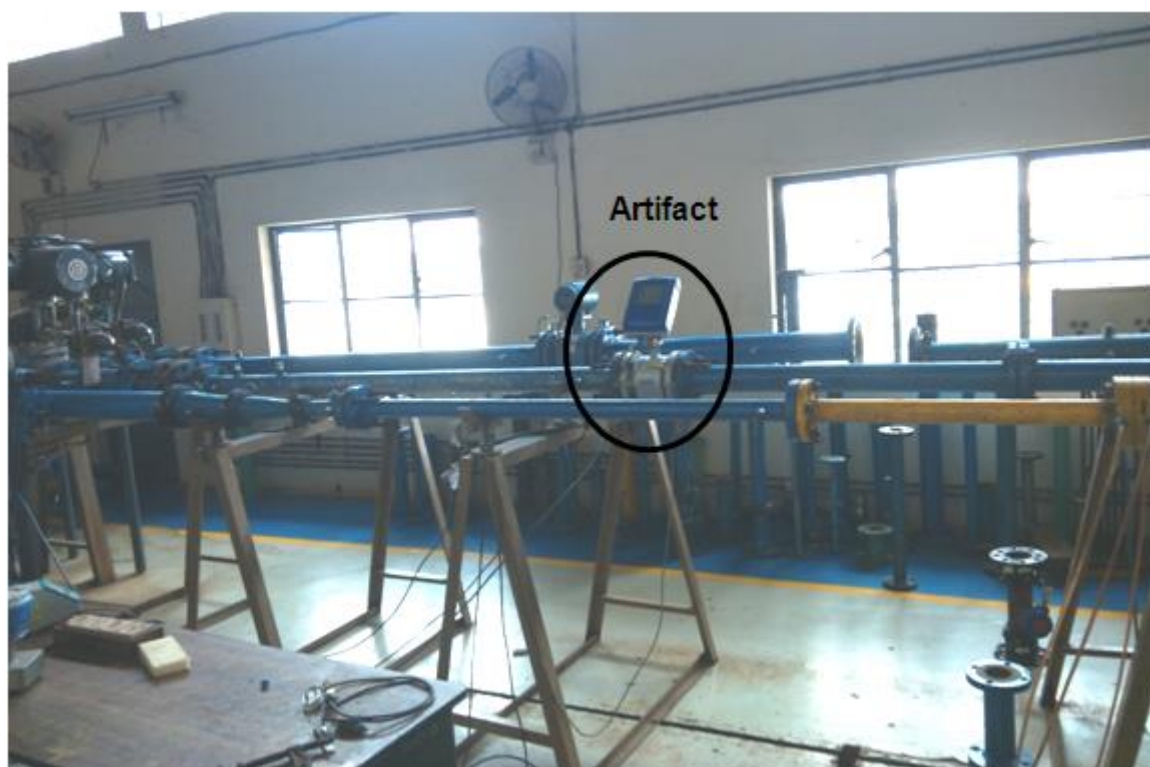
Figure 4.9: Photograph showing NPLI electromagnetic flowmeter installed at FCRI WFMS.
