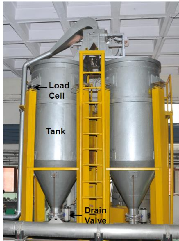
Figure 3.7: Weighing systems of new WFMS.
