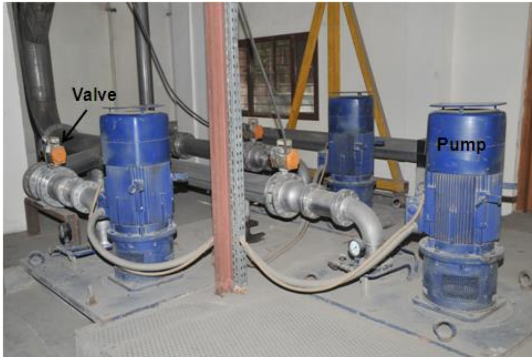
Figure 3.3: Pumps and manifold valves of New WFMS.
