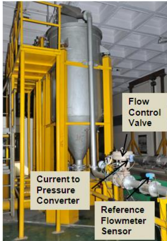
Figure 3.11: Photograph showing reference flowmeter and flow control valve.
