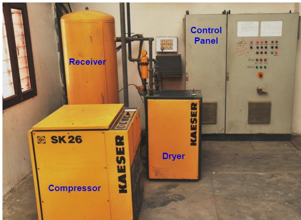
Figure 3.5: Air compressor system for new WFMS.
