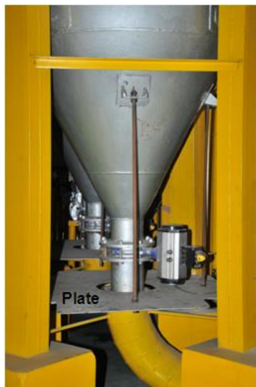
Figure 3.8: Plates and drain valves connected with the weighing systems.
