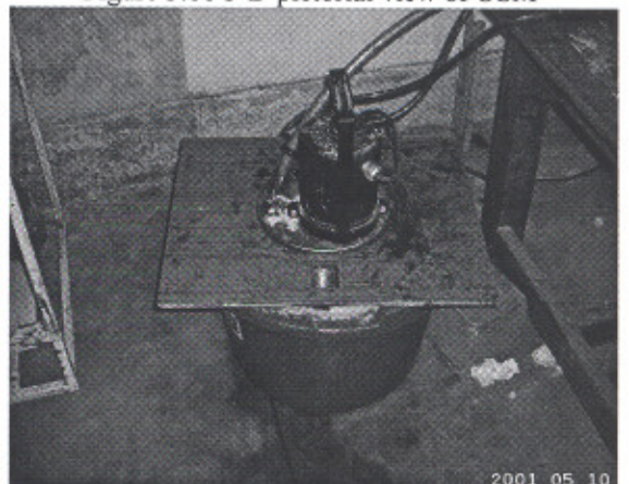
Figure 3.68 Pump for re-circulating slurry
