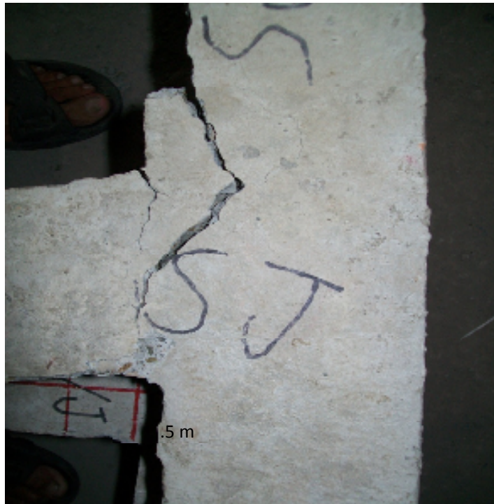
Plate 3.7 Crack Pattern of Joint 1 (100% damage)
