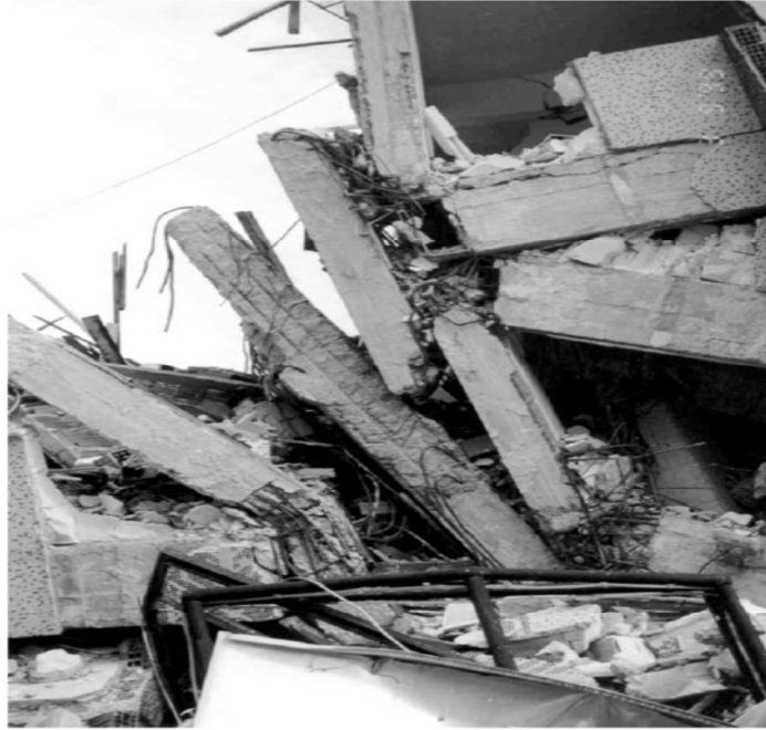
Plate 1.2 Joint failures during the Kocaeli (Turkey) earthquake
