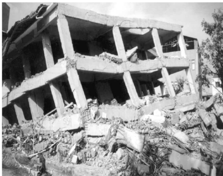
Plate 1.1 Beam-column joint shear failure
