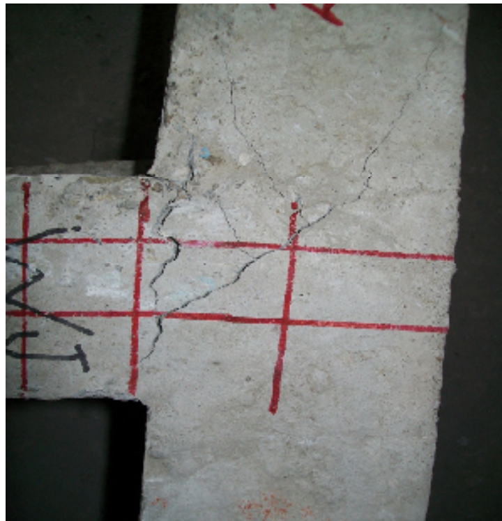
Plate 3.8 Crack Pattern of Joint 2 (100% damage)
