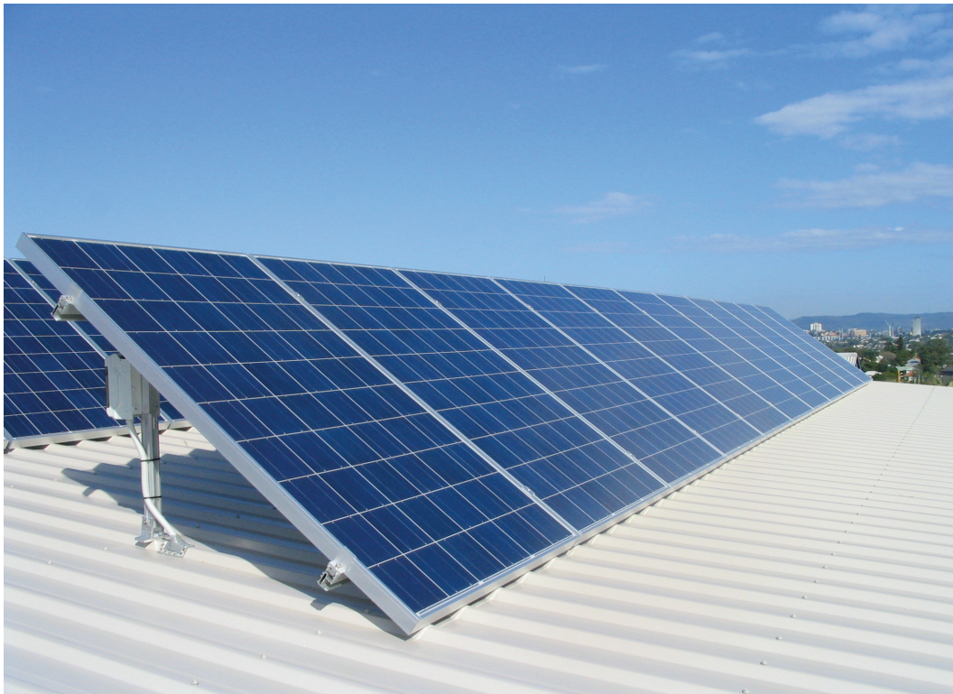
Fig. 3.6: Roof top PV panel [36].
