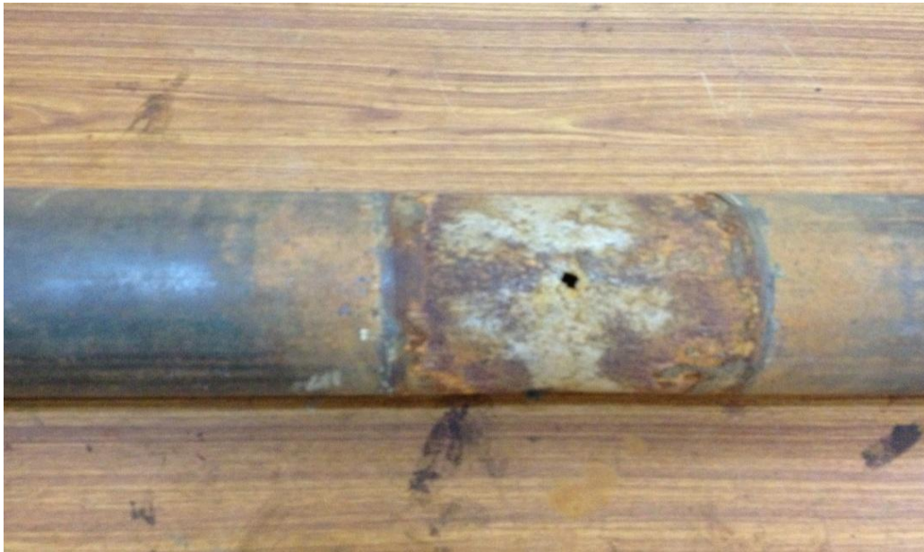
Figure 6.5: After corrosion hole formation in pipe
