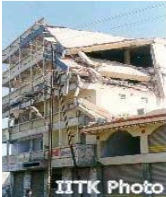
Fig. 1.1 Earthquake damage of RC building inter-story collapse in Bhuj, India (2001) (Sasmal, 2009).
