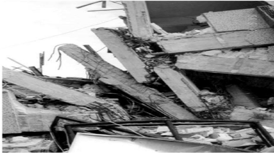
Figure 1.3 Joint failures during the Kocaeli (Turkey) earthquake (Ghobarah et al; 2002).
