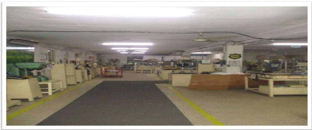
Figure 4.1.5: LED installation with proper Layout
