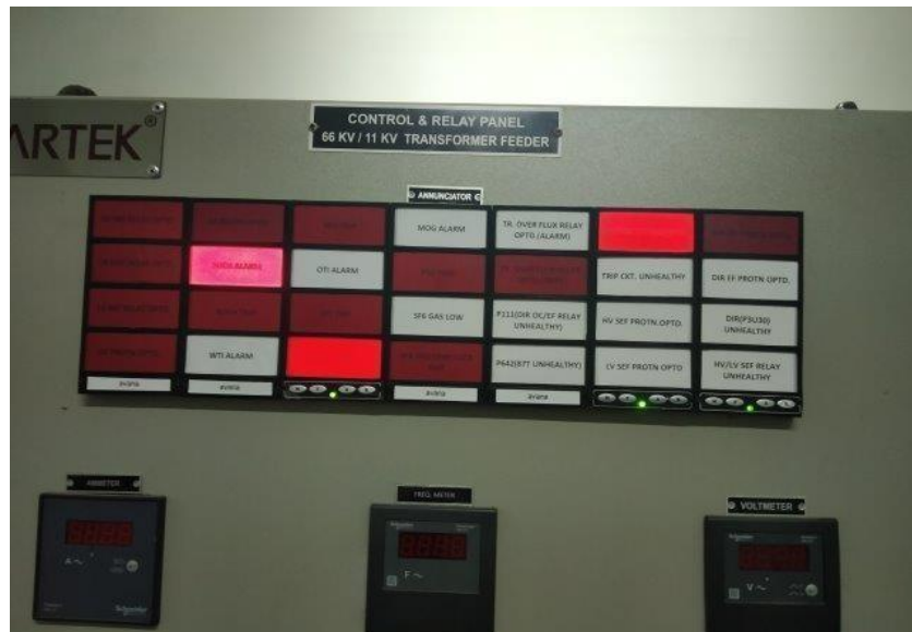
FIG.1.5: CONTROL AND RELAY PANEL
