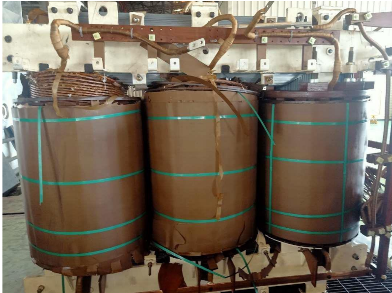
FIG.2.2: WINDING OVERVIEW AFTER SHORT CIRCUIT
