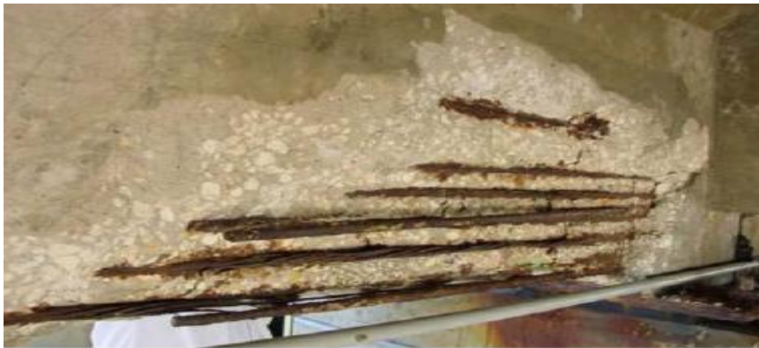
Fig. 4.3 Corrosion Damage to a concrete beam
