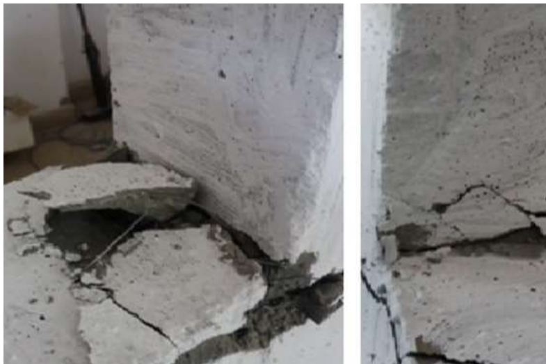
Figure 4.1 (d): Cracks formation at joint intersection. Figure 4.1 (e): Cracks formation at other side of joint.
