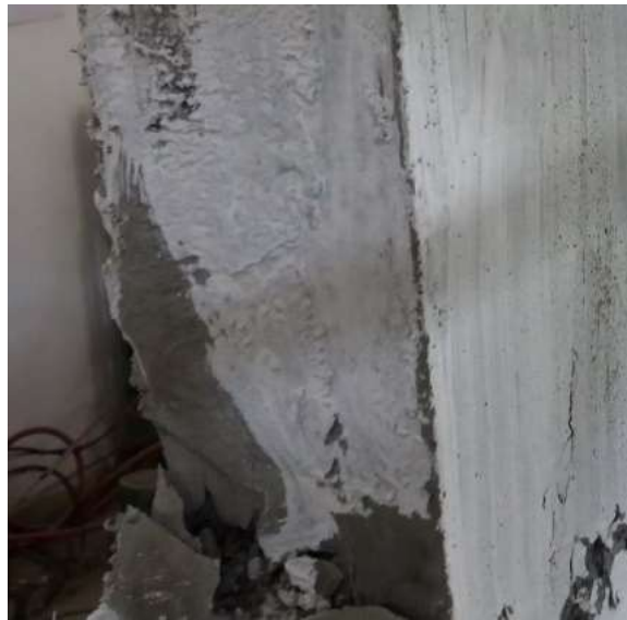
Figure 4.8 (d): Cracks after retrofitting.
