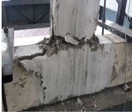
Figure 4.8 (c): Separation of HPFRCC layer from hardened concrete in RS3.
