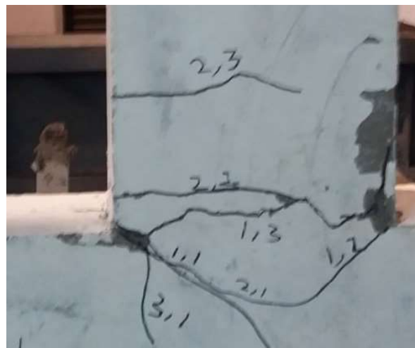
Figure 4.8 (b): Cracks propagation in specimen S3.
