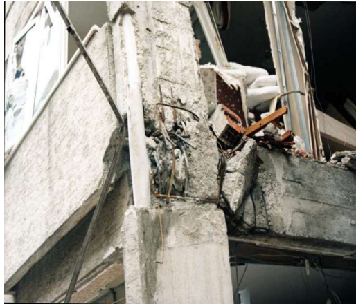
Figure 1.4: Damage of joint in an earthquake (1999 Kocaeli, Turkey)
