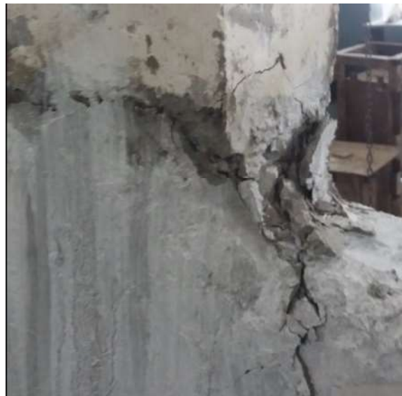
Figure 4.7 (c): Cracks formation after retrofitting for specimen RS2.
