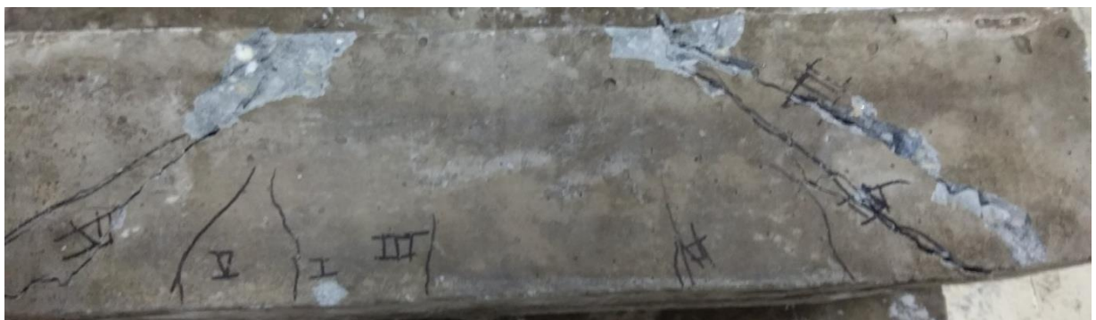
Figure 4.36 Cracks in G4 (2) of grade M30 beam at ultimate load 80.2kN
