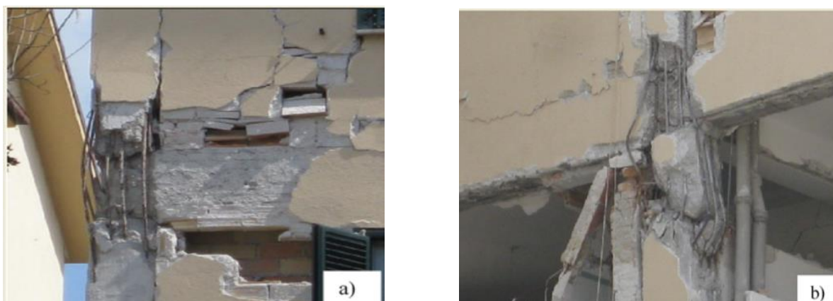
Figure 1. 2 Typical Beam Column Joint Failure (Beschi et al. 2015)
