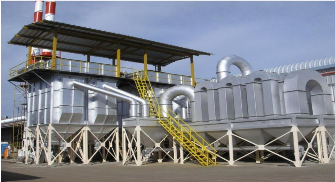
Figure 3.4 Waste Lead-acid batteries recycling plant (Recycling Plant)
