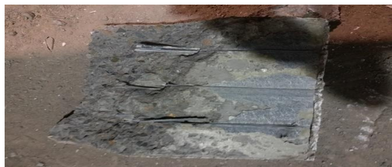
Fig.4.21 Separated Concrete Part After Failure
