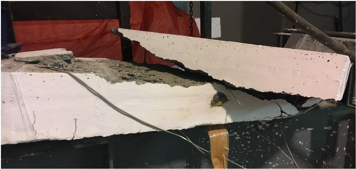
Fig.4.49(a) Actual Cracked Specimen at Failure
