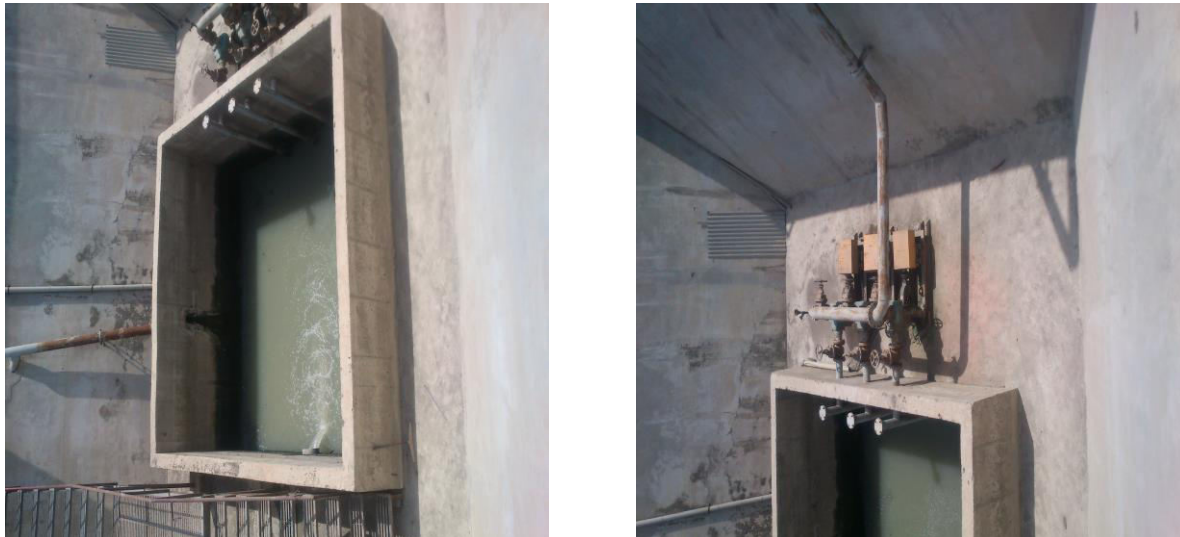
Fig 3.1 Raw sewage sump and raw sewage pumps
