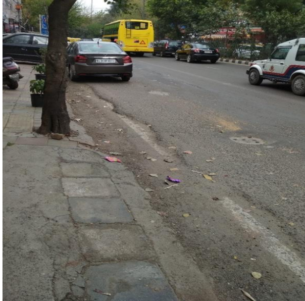
Figure 3.3: The existing condition near SDMC public co-educational school
