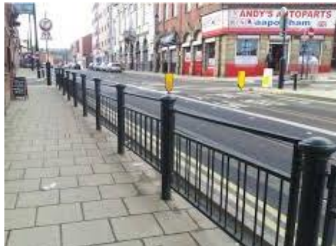
Figure7.3 : Sidewalk with Guardrail having visibility gap for school going children at 2 meters height
