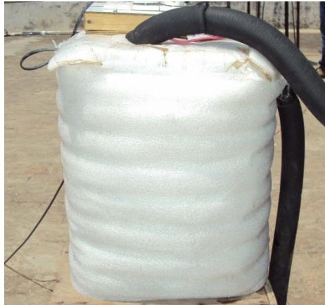
Figure 6.7 Storage Tank in PTC
