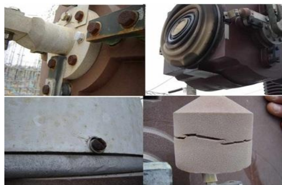
Figure 2.4 IT Visual inspection components (Clockwise direction: Terminals, membranes, bolts and spark gaps)
