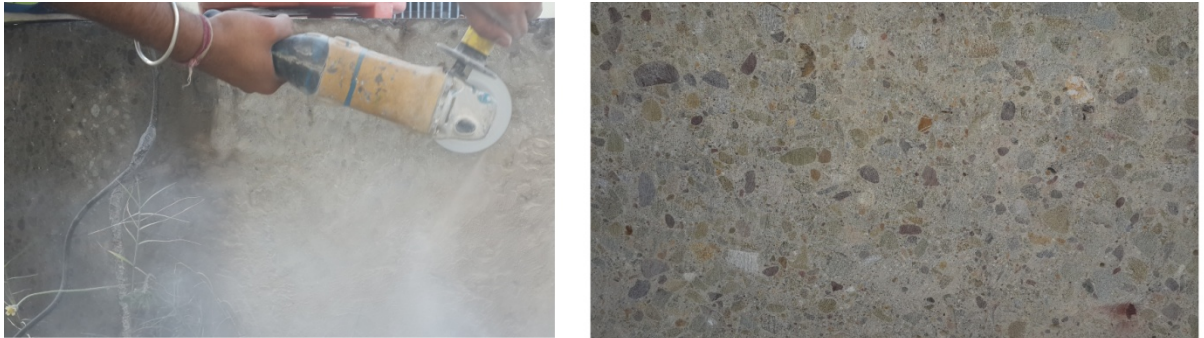
Fig 3.7 Grinding of the Beam with Hand Grinder and Exposed Aggregates after Grinding
