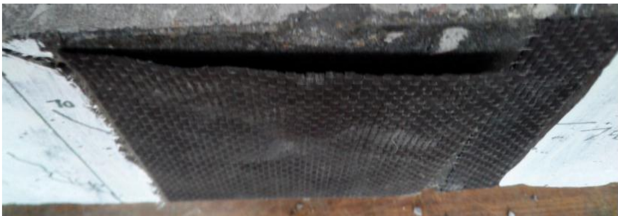
Figure 4.17 – Debonding of CFRP U-wrap in strengthened beam SB-06
