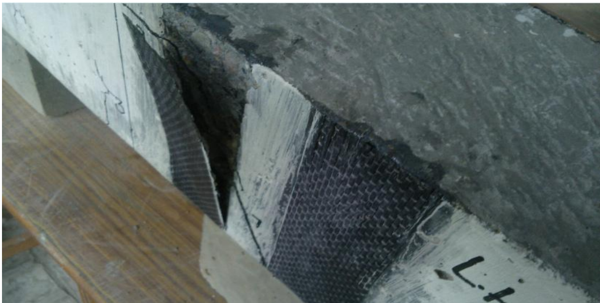
Figure 4.13 – Debonding of CFRP U-strip in strengthened beam SB-04
