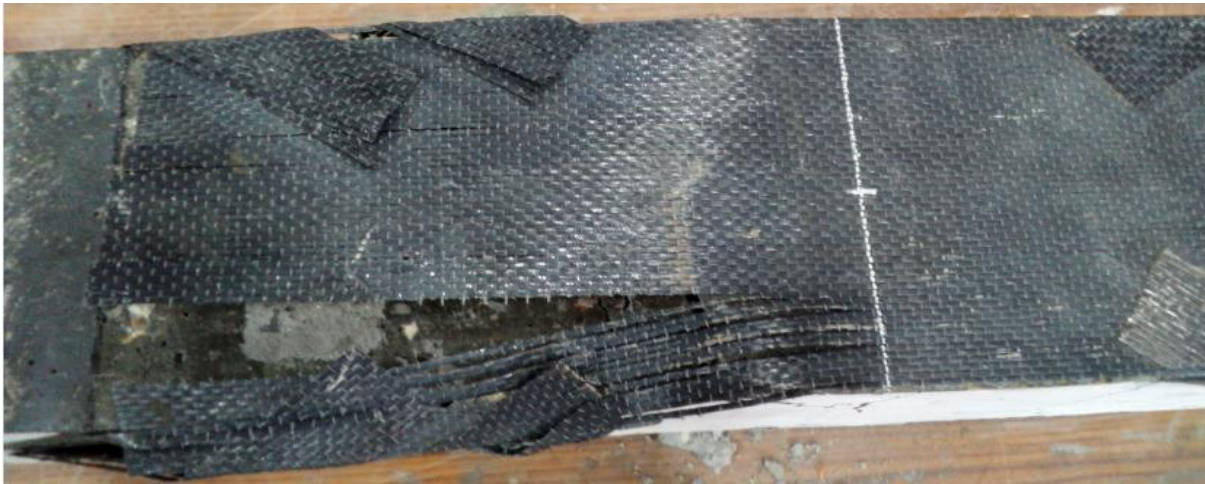
Figure 4.25 – Plate End Debonding in strengthened beam SB-10
