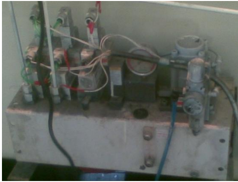
Figure 7.2: Power source of hydraulic clamping[Crompton Greaves, Ahmednagar]
