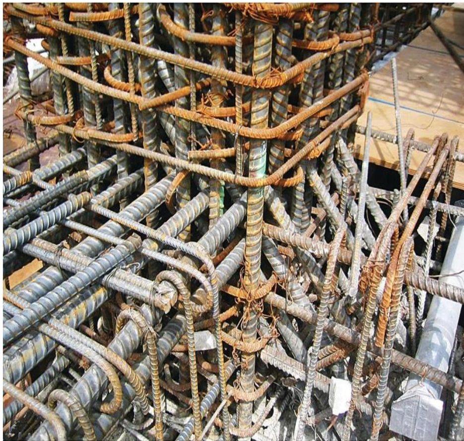
Figure 1. 1 Congestion in the beam-column joint due to the use of conventional bars (Bashandy 1996)
