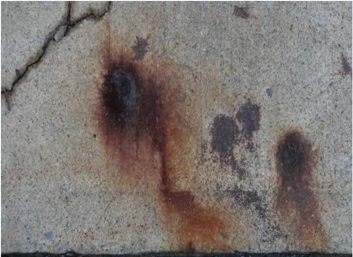
Fig. 1.3: Rust stains on concrete surface due to carbonation induced corrosion
