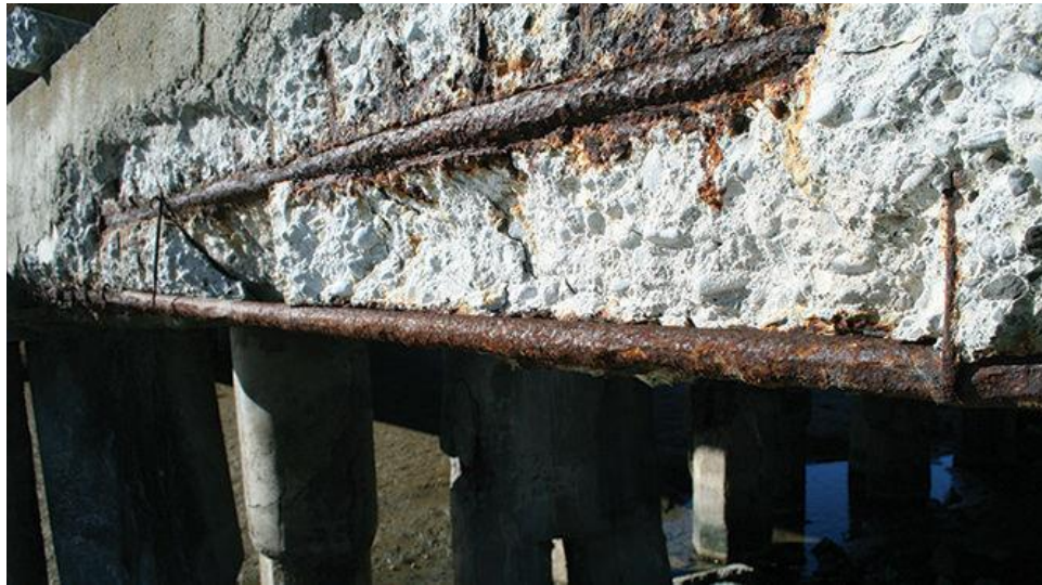
Fig.1.1: Spalling of concrete cover due corrosion of rebars
