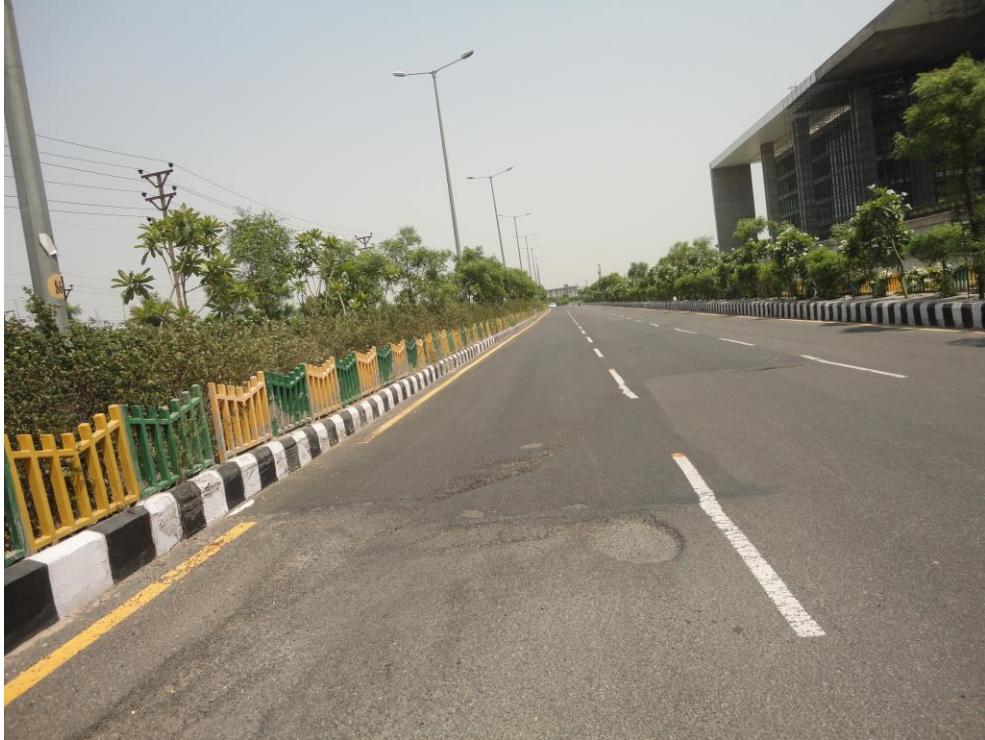
Plate 3.3: View of Pothole and Ravelling on J.P. Associate Office to Shani Temple
