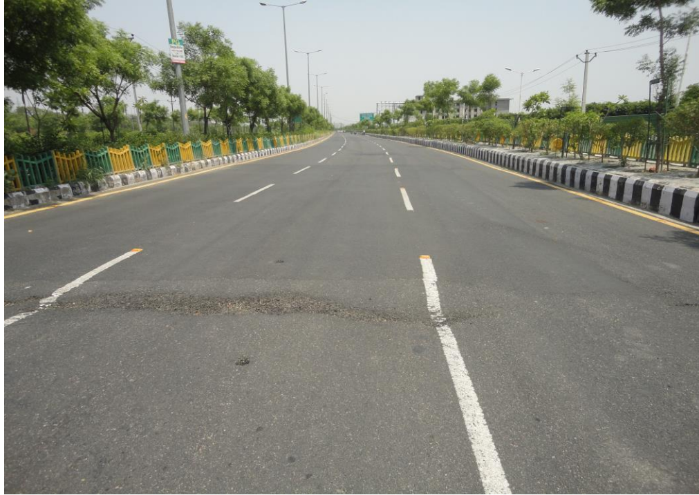
Plate 3.1: View of Slippage on Shani Temple to J.P.Associate Office
