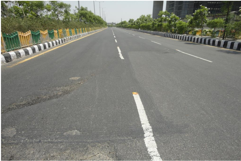
Plate 3.4: View of Patching and Ravelling on J.P. Associate Office to Shani Temple
