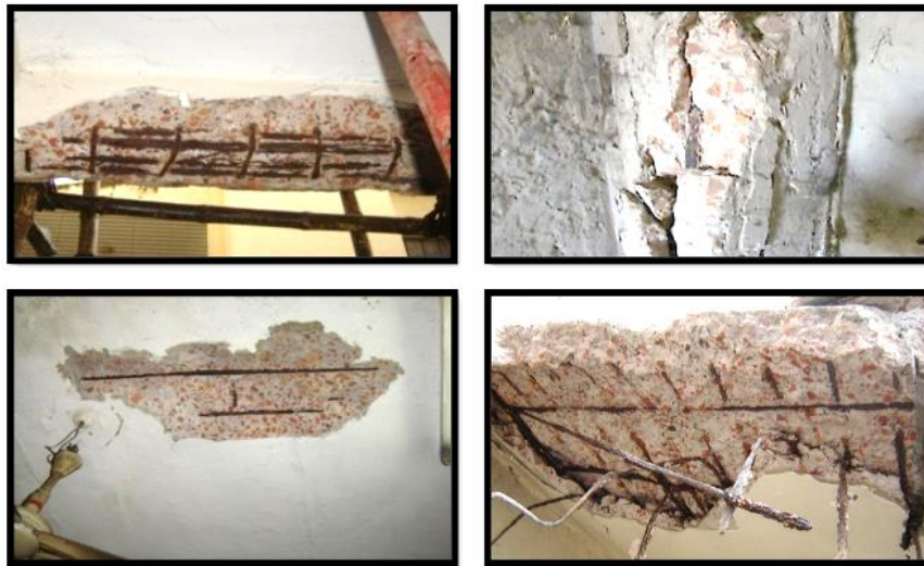
Figure 2.5 Structures corroding due to carbonation (Uddin et al., 2013)
