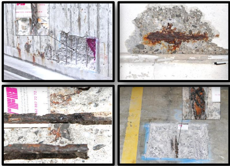
Figure 2.4 Structures corroding due to chloride ions' ingress (Bisschop, 2016)
