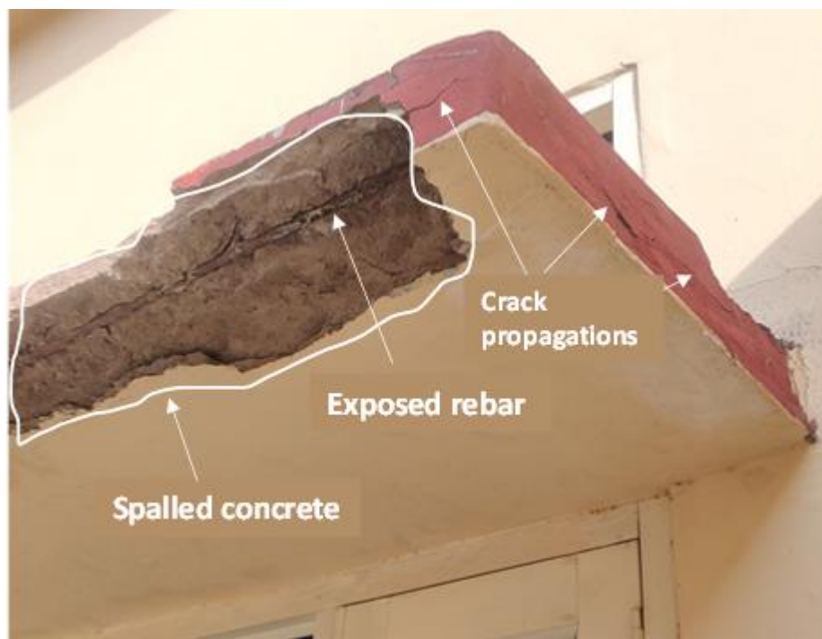
Figure 6.6 Observations from visual inspection of RC slab to be repaired
