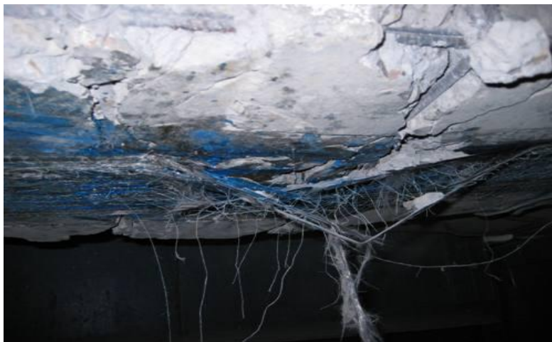
Fig 4.4 Debonding of sheet from the beam
