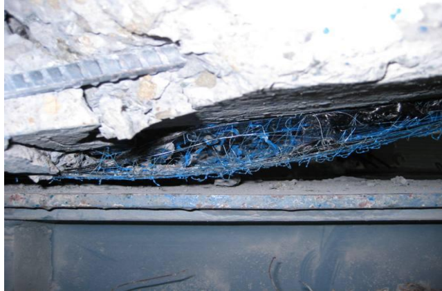
Fig 4.8 Debonding of Fiber sheets from the beam
