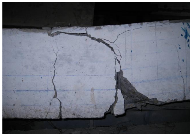
Fig 4.9 Failure pattern of beam retrofitted with double layer prestressed fiber sheet
