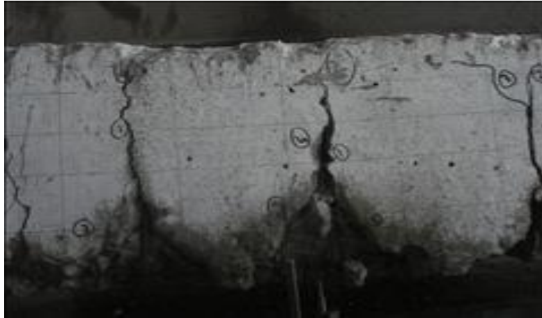
Fig 4.5 Bending cracks and spalling of concrete
