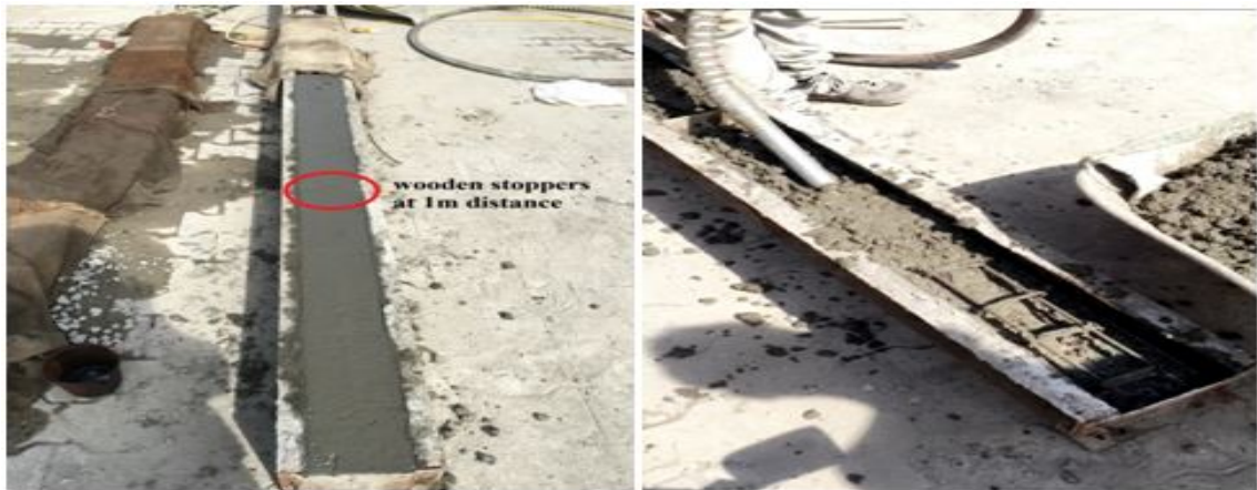
Figure 3. 3 : Figure showing filling of concrete in mould and vibrating with needle vibrator
