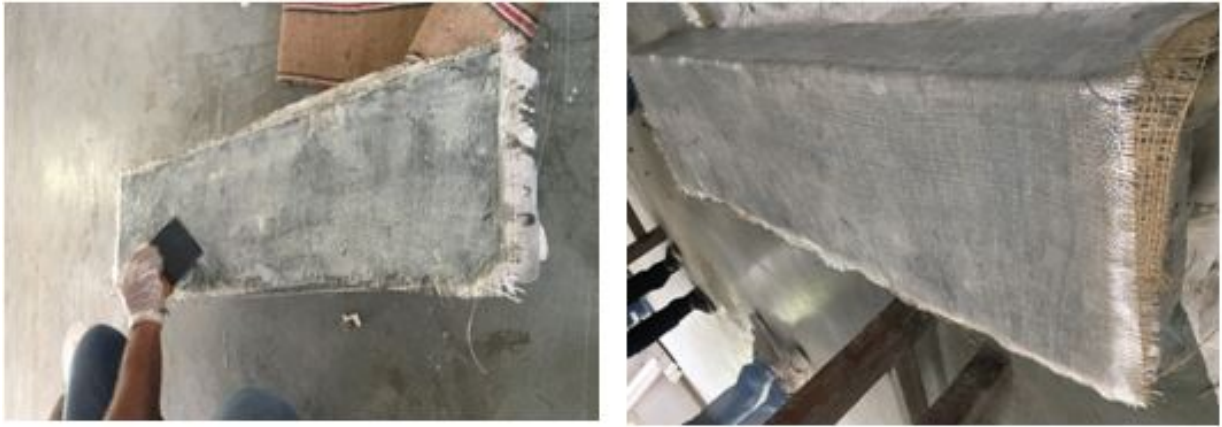
Figure 3. 6 : Retrofitting of beams with side and U wrapping technique by applying epoxy over jute and glass fabrics
