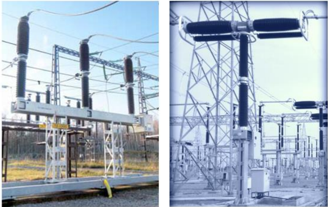
Figure 2: Circuit breaker for 145kV (L) and 420 kV (R)
