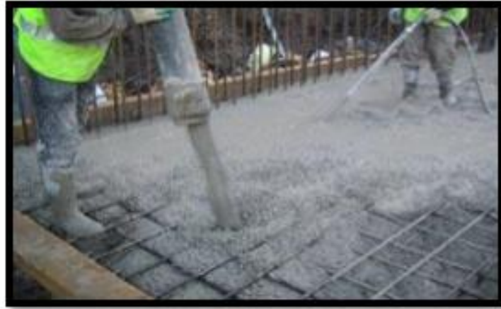
Figure 1.4: Showing that the workability is more and pumping is easier (Suresh, D. et. al, 2015)
