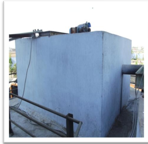
Chemical Dosing Tank
