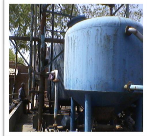
Pressure sand Filter & Activated Carbon Filter
