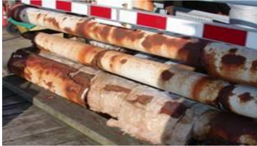
Figure 1.12 High temperature corrosion (Source: amteccorrosion)
