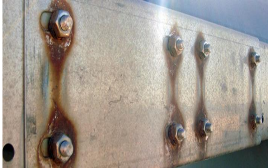
Figure 1.8 Galvanic Corrosion (Source: steelfabservices)
