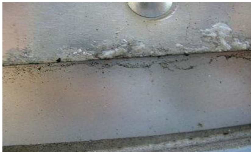
Figure 1.7 Filiform Corrosion (Source: airforums)
