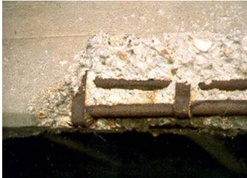
Figure 1.2 Carbonation induced corrosion on concrete (Source: corrosionengineering)
