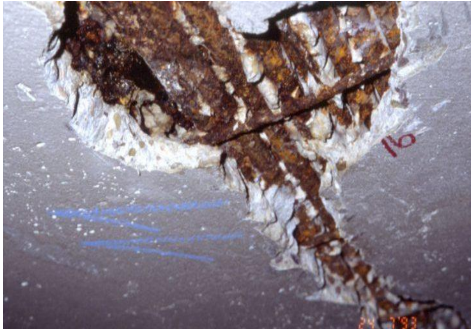
Figure 1.3 Chloride induced corrosion on concrete (Source: civilengineeringforum)
