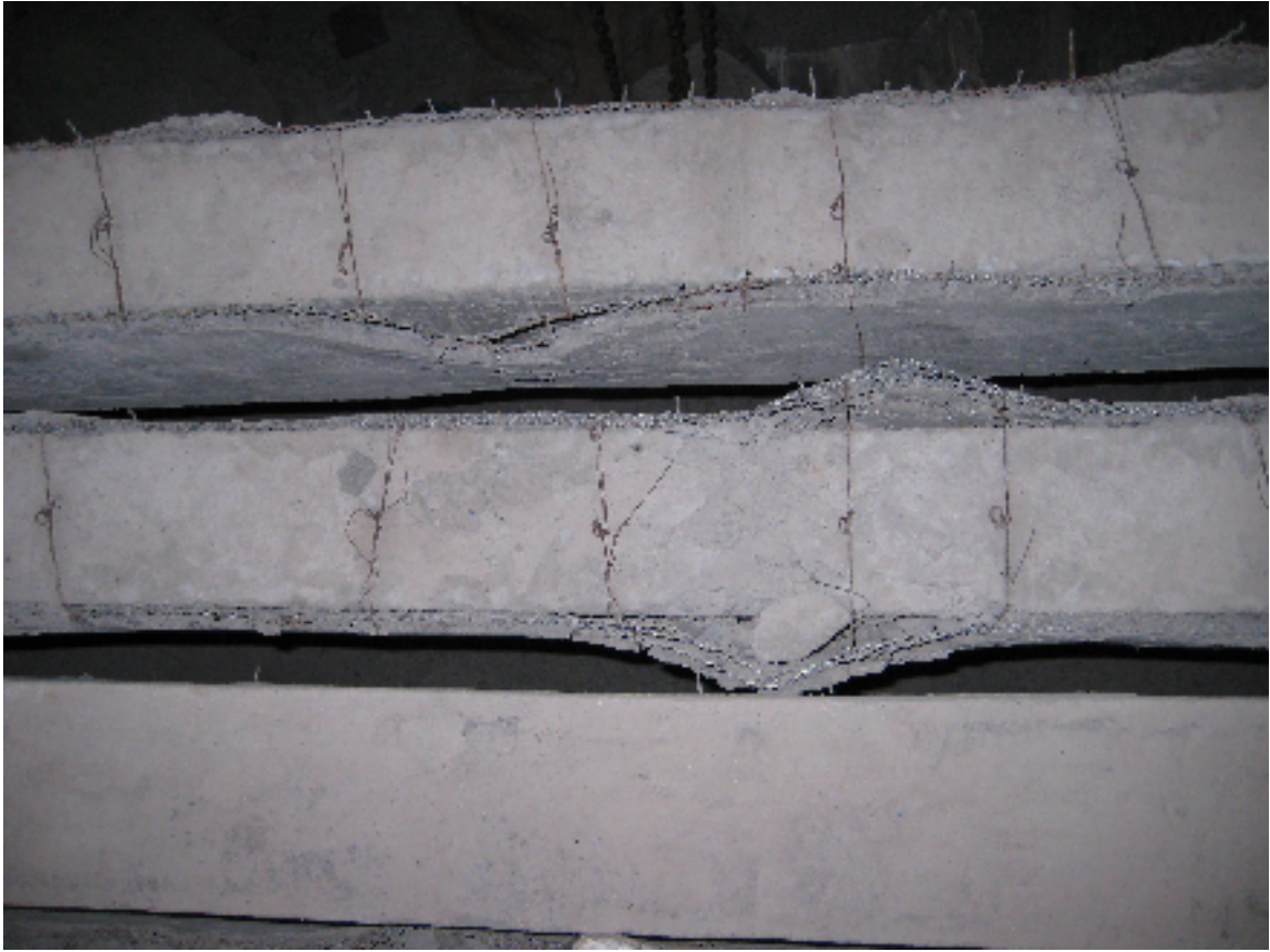
PLATE 3.9: FAILURE OF BEAMS
