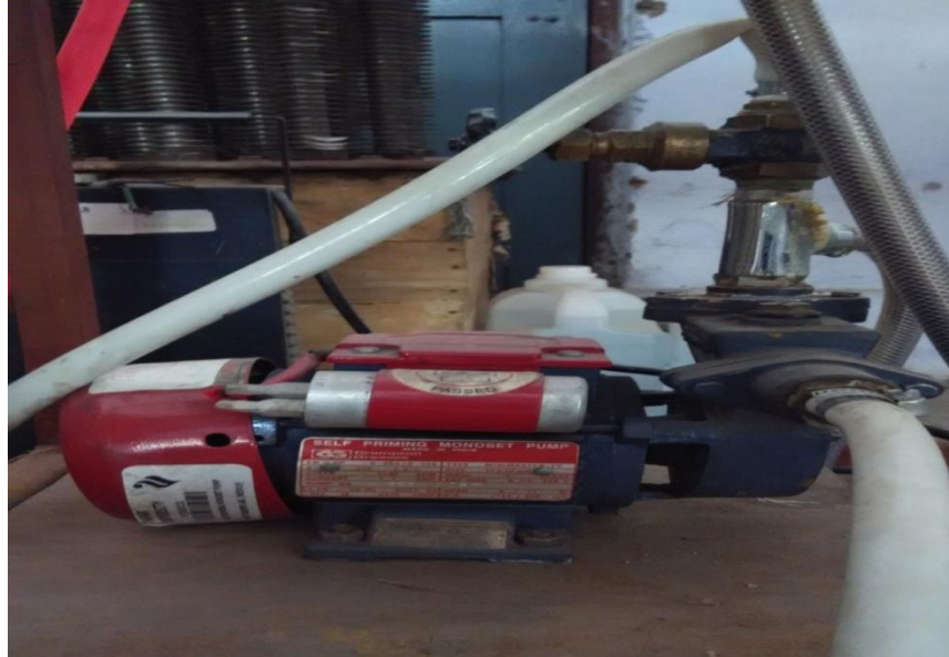
Figure 4.6 Centrifugal pumps used for circulating fluids
