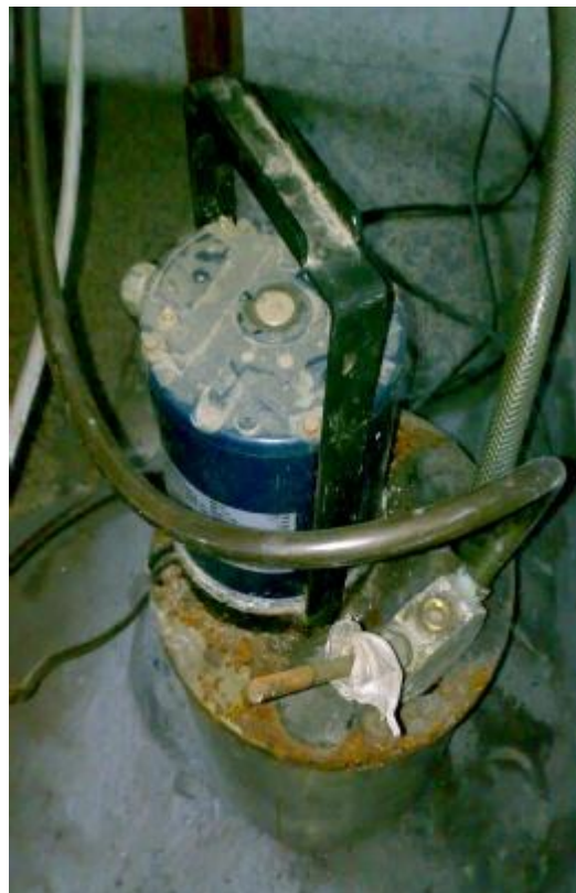
Fig: 7.5 Pump for Re-circulation of Abrasive slurry
