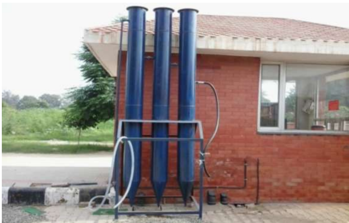
Figure 4.20: 3-stage multi-grade up-flow roughing filter installed
