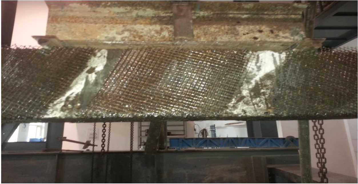
Figure 4.12 Failure and Crack Pattern of Beam Strengthened with Inclined Strips on center
