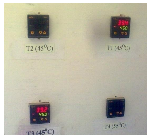
Fig. 4.19 Temperature display panel with controller
