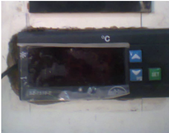
Fig.5.16: Digital temperature controller
