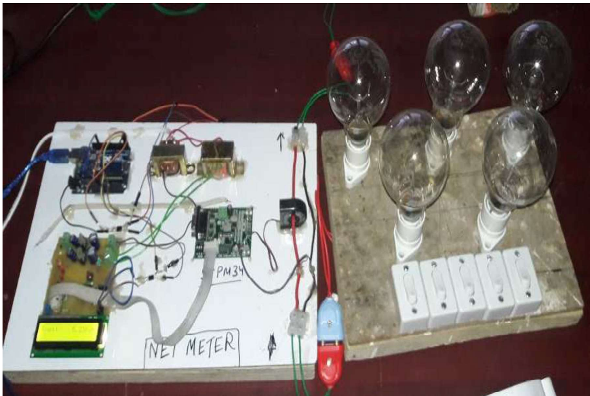
Figure 5.14: Experimental setup for net energy meter demonstration
