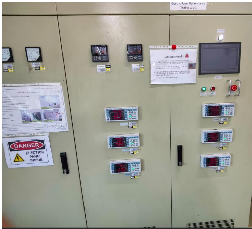
Figure 3.23 Electric Panel for performance handling and measurement
