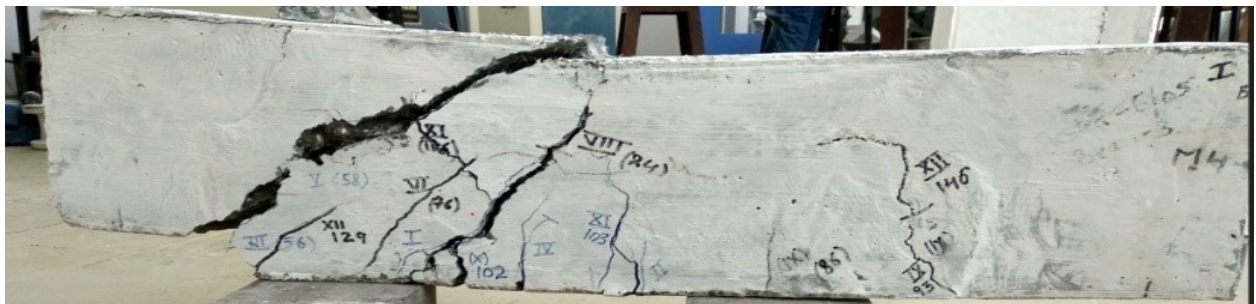
Fig 4.17 Cracking pattern of beam repaired with Mix M4
