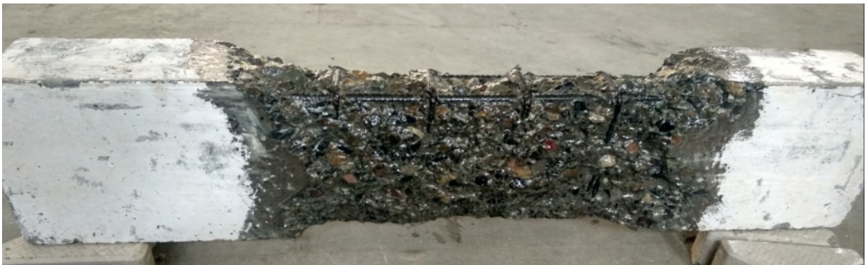
Fig 3.10 Damaged beam after application of epoxy
