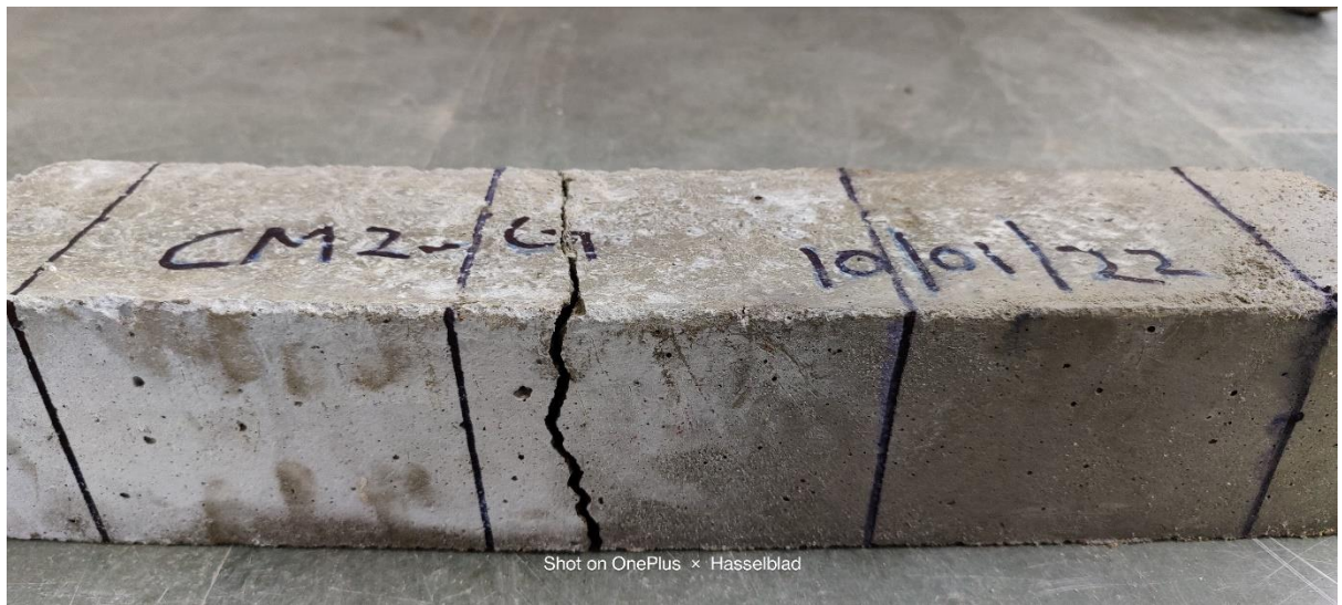
Figure 4.12 Side view of crack pattern in beam specimen used in present study
