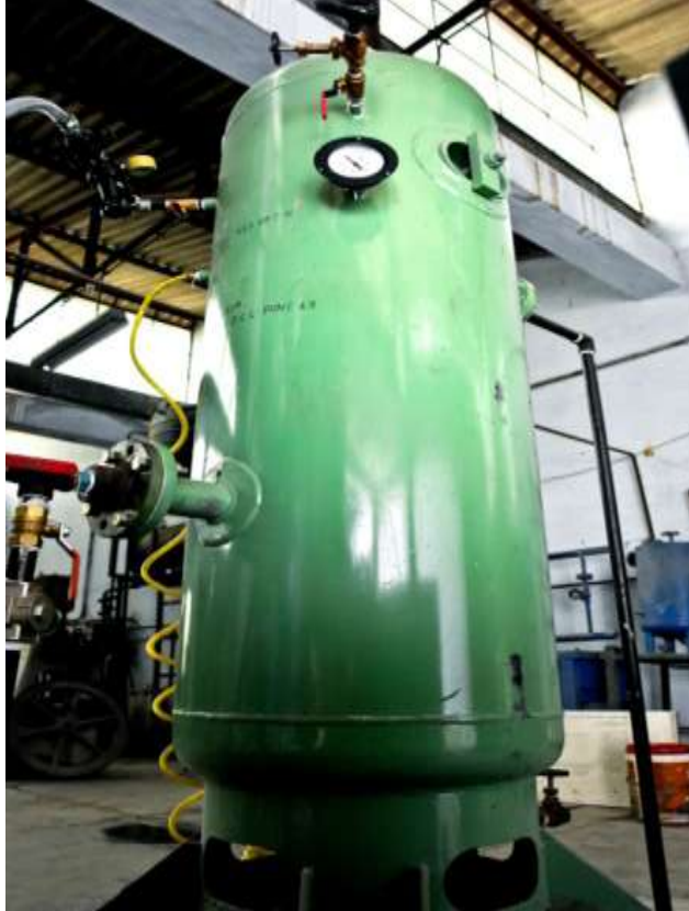
Figure 3.3 Air Receiver Tank in TU laboratory
