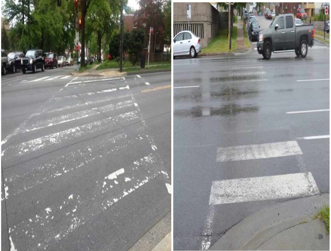
Figure 9.4 Showing Faded Marking Conditions
