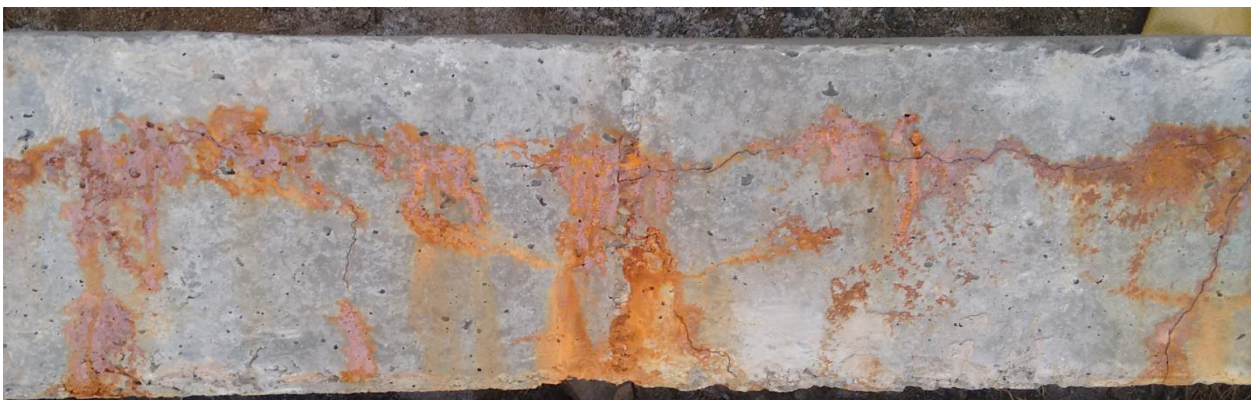
Figure 4.2 Cracks on left face of C-30
