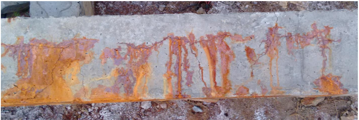
Figure 4.4 Longitudnal and tranverse cracks at right face of C-40
