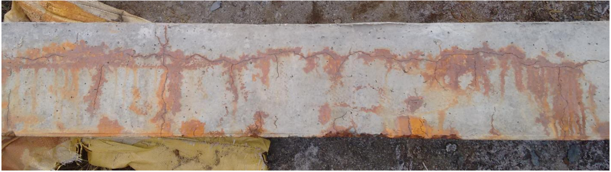
Figure 4.3 Longitudnal and tranverse cracks at right face of C-30
